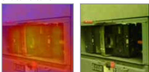
Normal operating temperature on mission critical breaker
